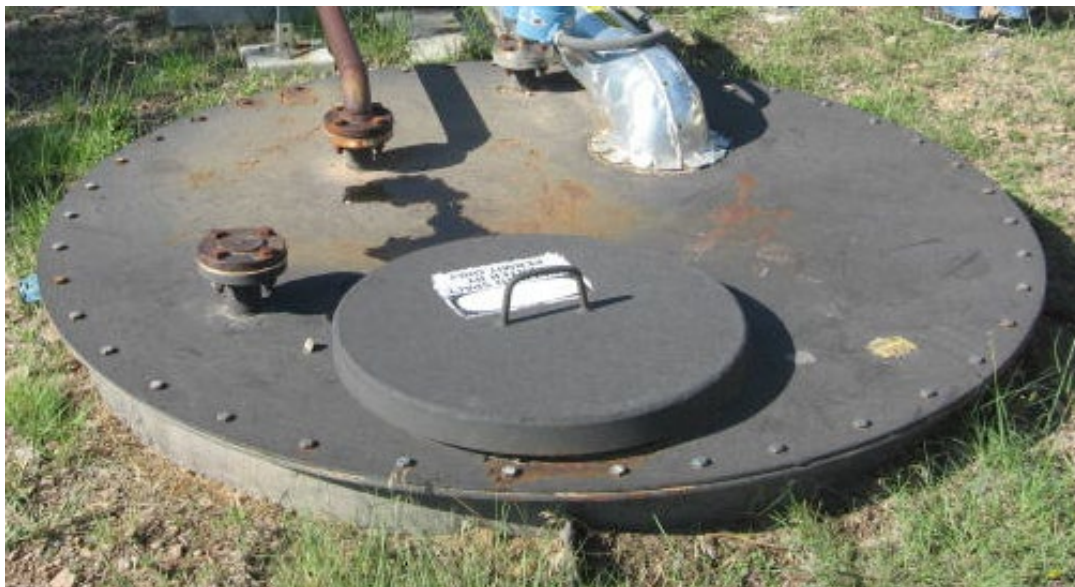
Photograph - NPDES-05A055-18-007 HEWTF - Underground Storage Tanks
