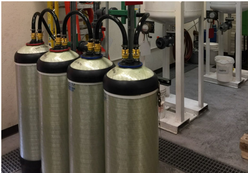
Photograph - NPDES-05A055-18-011 HEWTF - Ion Exchange Tanks
