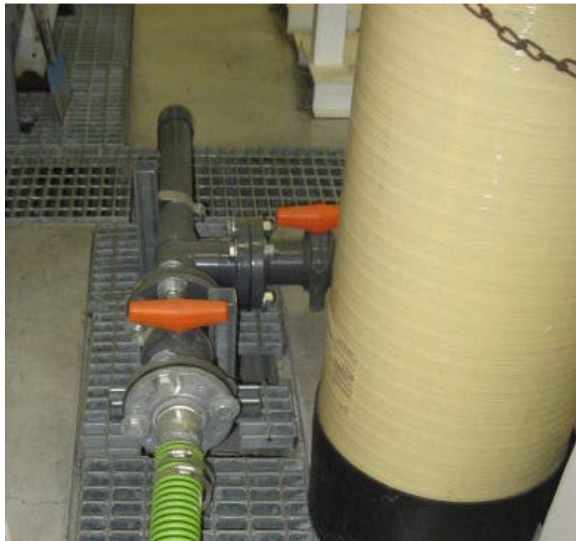
Photograph - NPDES-05A055-18-003 Outfall 05A055 - Condition at Hose Connection for Discharge to the Outfall
