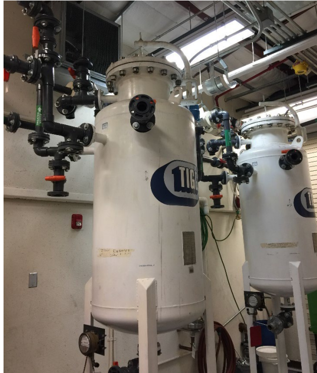
Photograph - NPDES-05A055-18-010 HEWTF - Activated Carbon Filter Tanks
