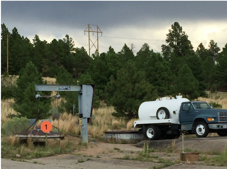
Photograph - NPDES-05A055-18-005 HEWTF – Sand Filters and Tanker Truck
