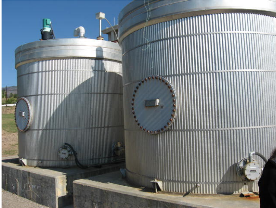
Photograph - NPDES-05A055-18-012 HEWTF - Post Treatment Tanks
