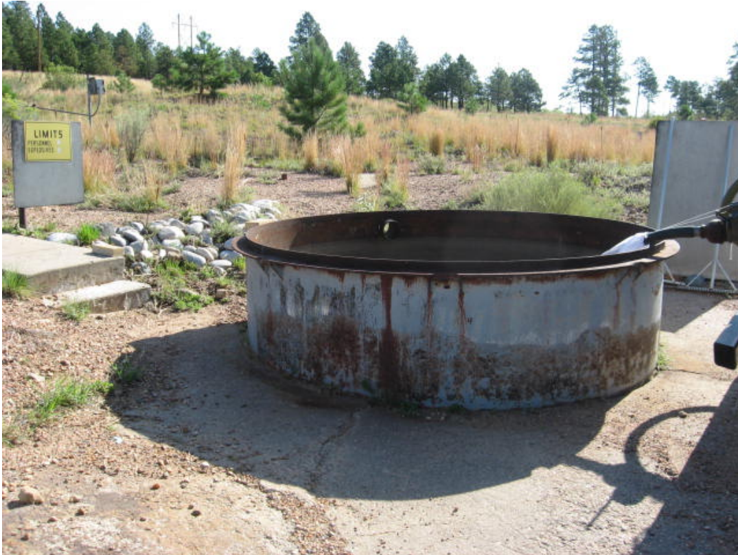
Photograph - NPDES-05A055-18-006 HEWTF – Sand Filter
