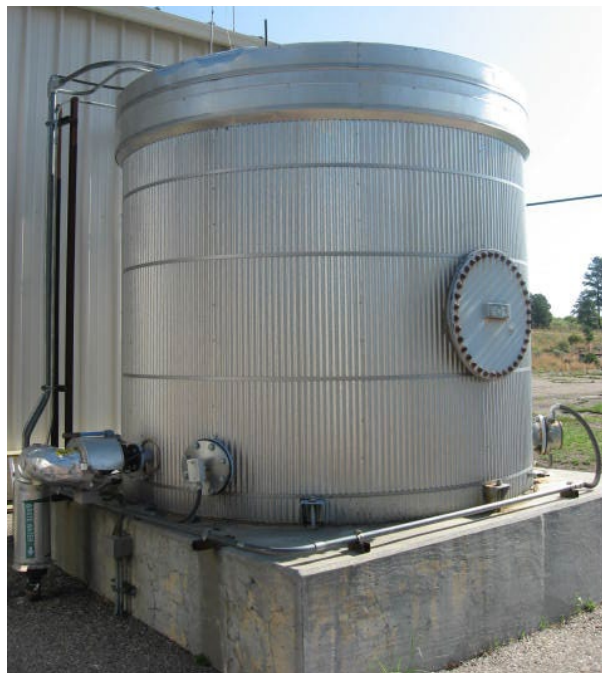
Photograph - NPDES-05A055-18-009 HEWTF - Equalization Tank
